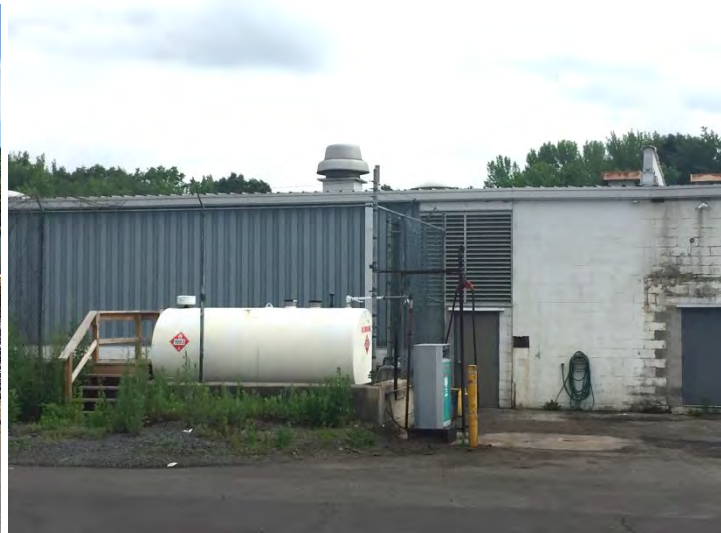
+/- 2,000 Gallon Diesel Fueling Station
